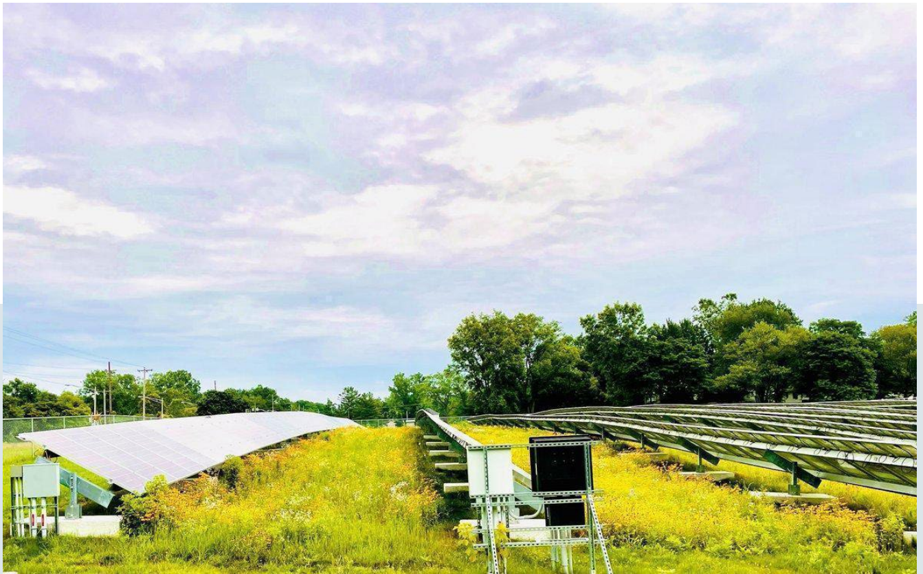
The East Lansing Community Solar Park.
